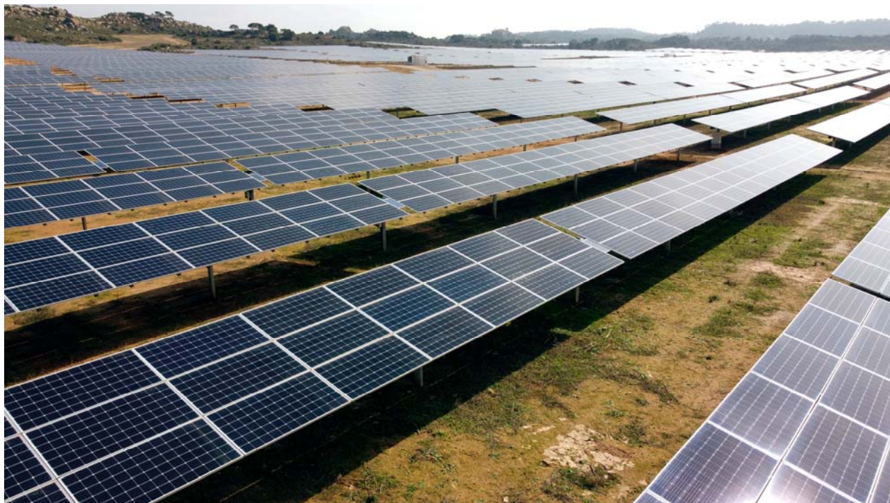
View of the solar plant Desafío Solar SLU
